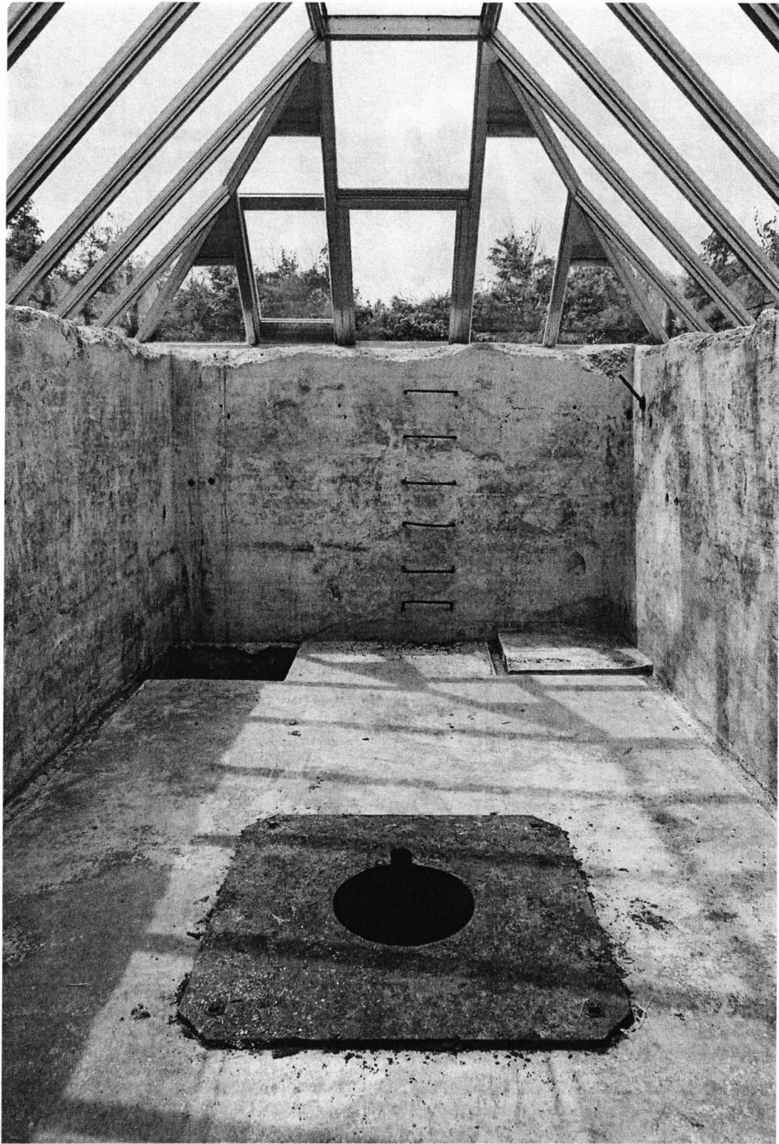
Here is a photo showing the interior of the loading pit taken in August 2005. Visible here is the hole in the rusted steel plate at the bottom where the hydraulic lift column was located. (Author)
